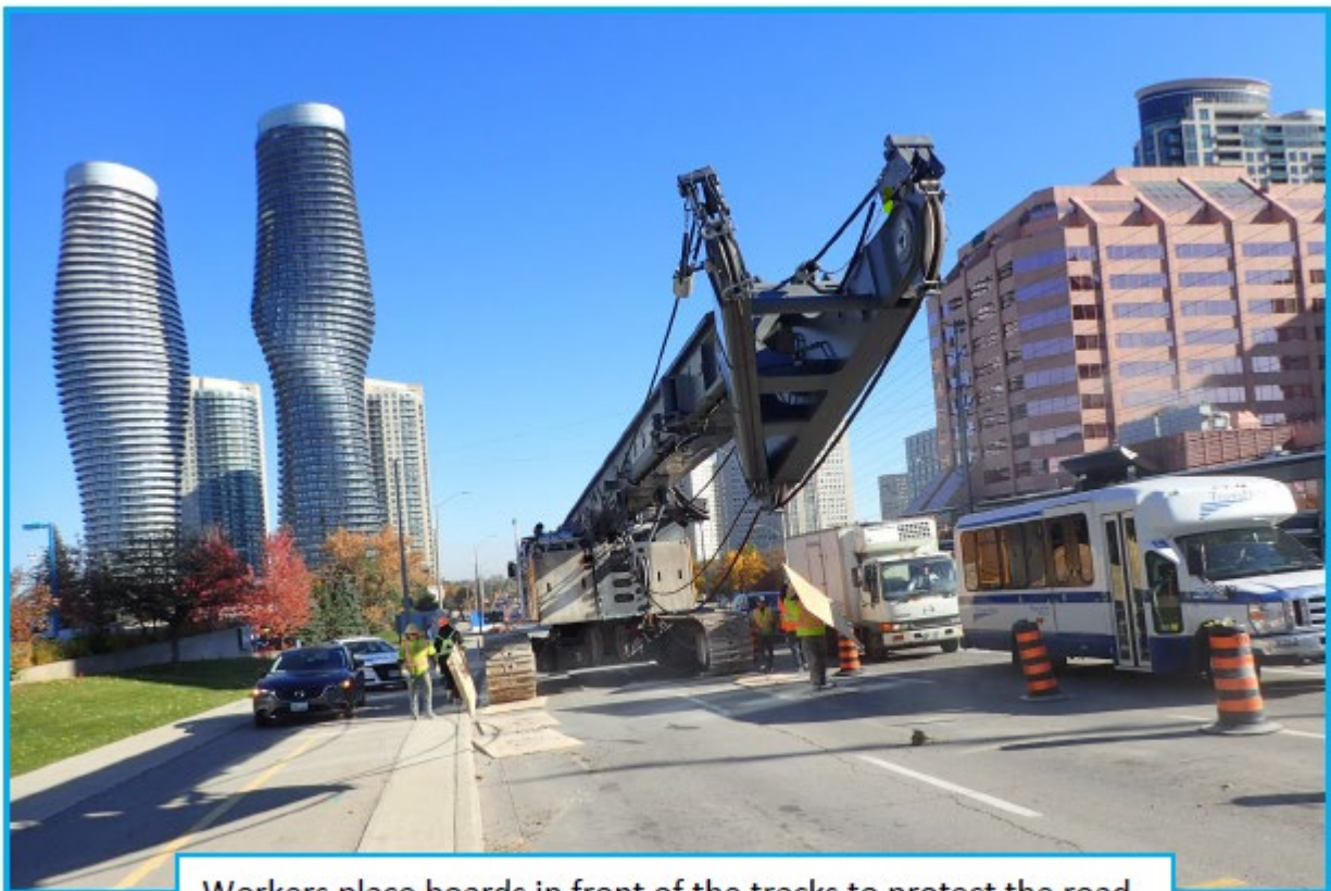
Workers place boards in front of the tracks to protect the road.
