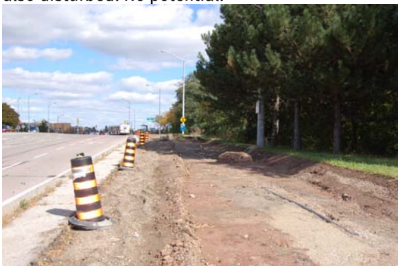
Plate 17: View northeast along Derry Road West. ROW is disturbed. No potential. Lands beyond ROW have potential. Require Stage 2 test-pit survey.
