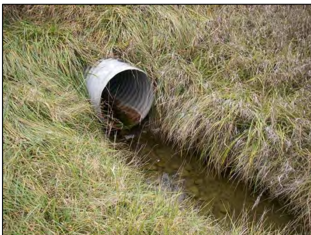
Downstream end of culvert facing upstream (west). Note channel definition and perched condition
