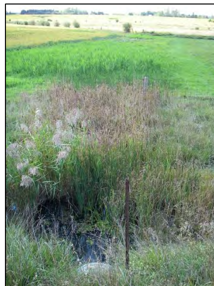
Downstream (west) end of culvert facing downstream. Note that watercourse vegetation had been cut
