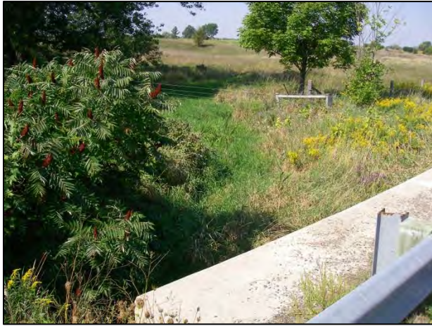
Salt Creek upstream (west) of culvert. Note fence and pasture in background
