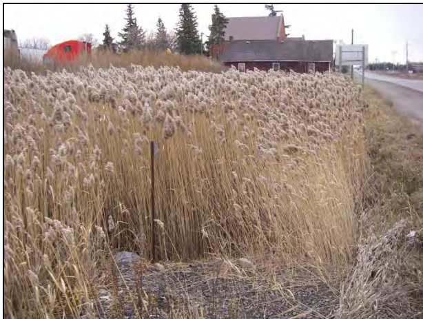
Facing downstream (southeast) at downstream end of culvert. Note culvert end is not perpendicular to road
