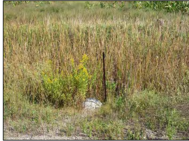
Upstream end of culvert facing east showing small patch of cattails with corn field in background
