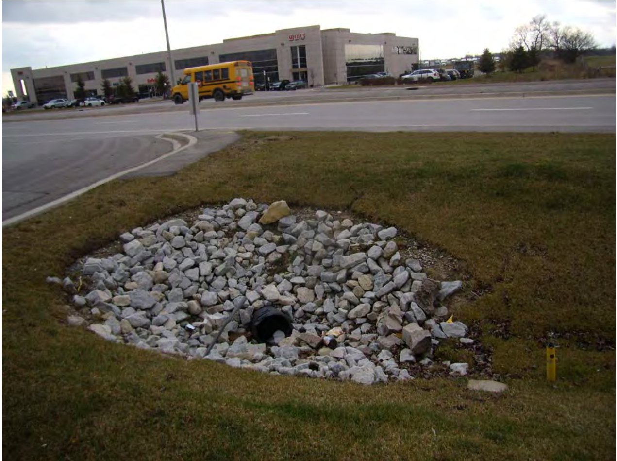
Crossing 1 recently replaced with ditch pipes (either side of the road) connecting to Airport Road storm sewer (Approximately 610m North of Mayfield Road)
