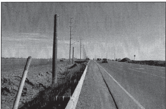
Plate 3: View to the northwest along the north side of Bovaird Drive at disturbed ROW due to widening of the intersection.
