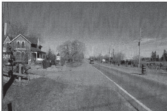
Plate 4: View to the northwest along west side of Mississauga Road at distributed ROW where additional shafts of sewer installations are to occur
