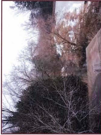
Figure 33: West Humber River Tributary and Large Box Culvert West of Dixie Road (looking southwest)
