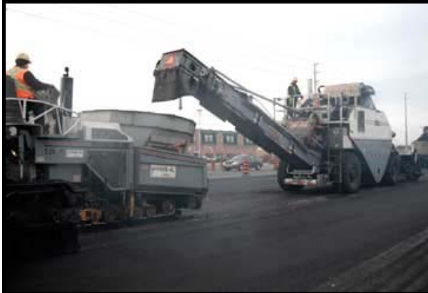
Available Physical Infrastructure
