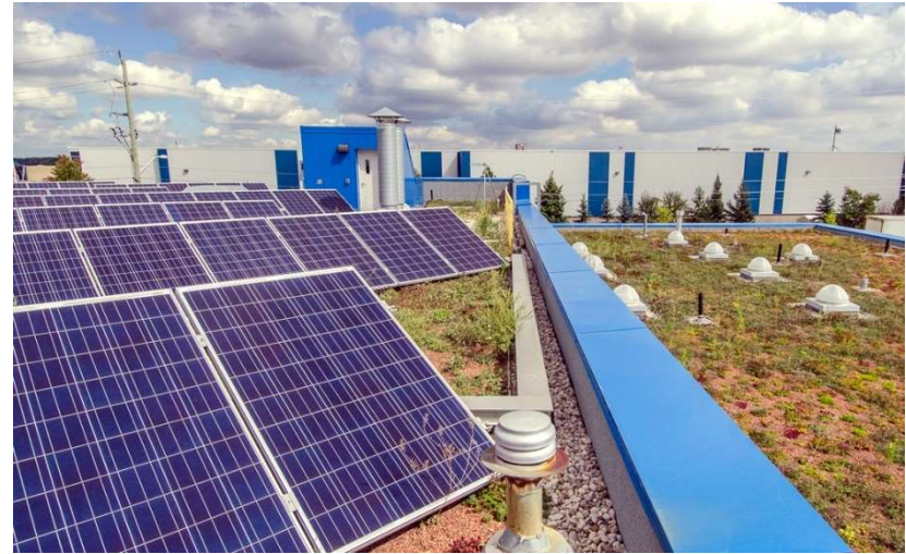
Solar panels on a green roof at the Heart Lake Community Recycling Centre
