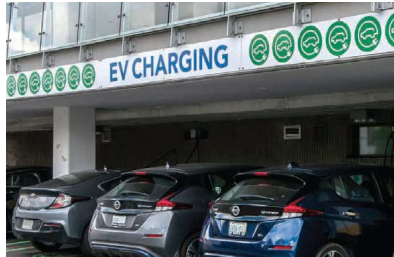
Electrical Vehicle (EV) charging at Regional Headquarters (10 Peel Centre Dr.)
